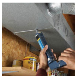
HVAC duct system
