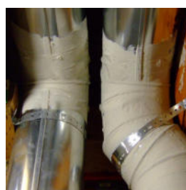
HVAC duct system
